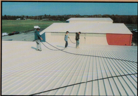
Final coat of Truco's Eterna-Seal® being applied resulting in a watertight membrane.
